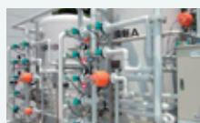
Lead discharge water recycling facility (ion-exchange towers)
