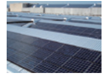
Toyota Motor Corporation Tsutsumi Plant (Japan) 2,000 kW
