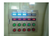
Control panel of the air-conditioning equipment
