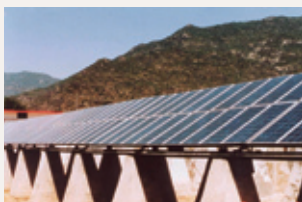
Solar power system donated to Kankoi Village
